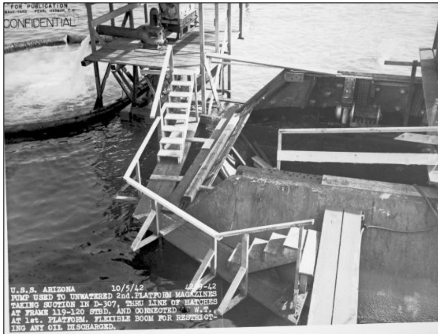
Figure 3.12. Pump and platform used to unwater second platform magazines, Space D-307, Frame 119-120, October 5, 1942 (USS Arizona Memorial Photo Archive).
